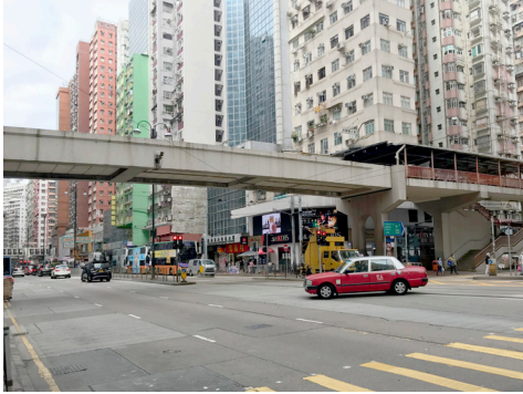
The pedestrian bridge populated by homeless people was set on fire in April, 2020. After the fire, the bridge section was barricaded and its cover removed.
